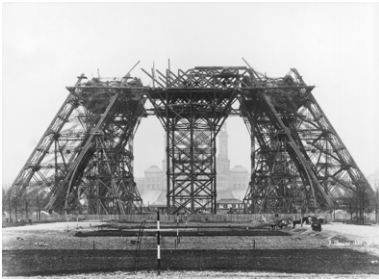
[Fig.4] The scaffolding on the first floor of the Eiffel Tower. January 1888. © Tour Eiffel Collection.
