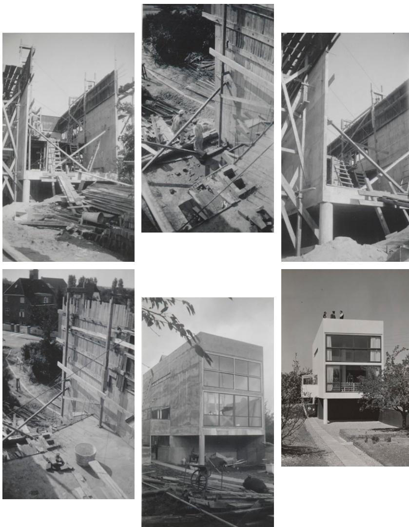
[Fig. 7-12] Images documenting the construction process of the house Anchersvej 6. Source: Royal Danish Library.
